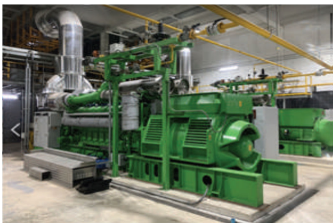
Exhibit 6: Gas engine and generator
