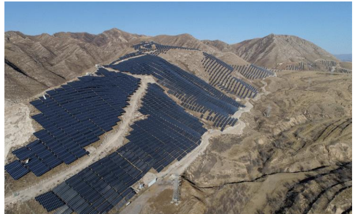
Exhibit 22: A photovoltaic power plant on the northern mountain of Caozhuangzi Village in the Xuanhua district of Zhangjiakou, Hebei Province, China
