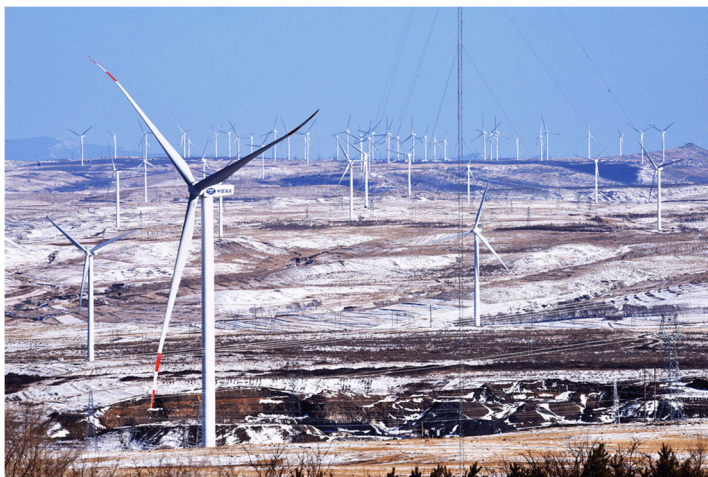
Exhibit 19: A wind farm in Hailiutu township in the county of Zhangbei in Zhangjiakou, Hebei Province, China
