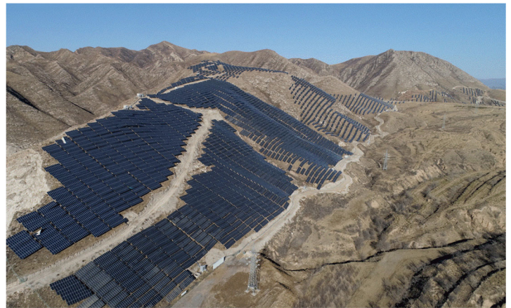
Exhibit 22: A photovoltaic power plant on the northern mountain of Caozhuangzi Village in the Xuanhua district of Zhangjiakou, Hebei Province, China
